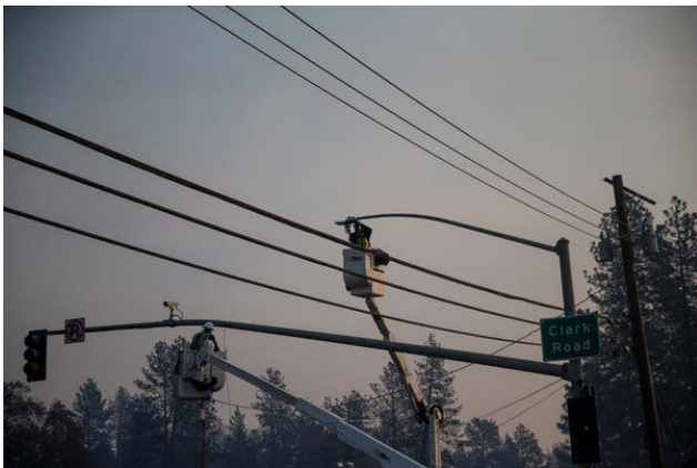
Crews working on power lines in the aftermath of last year’s Camp Fire in Paradise, Calif., which contributed to the bankruptcy filing by Pacific Gas and Electric. Credit Eric Thayer for The New York Times
