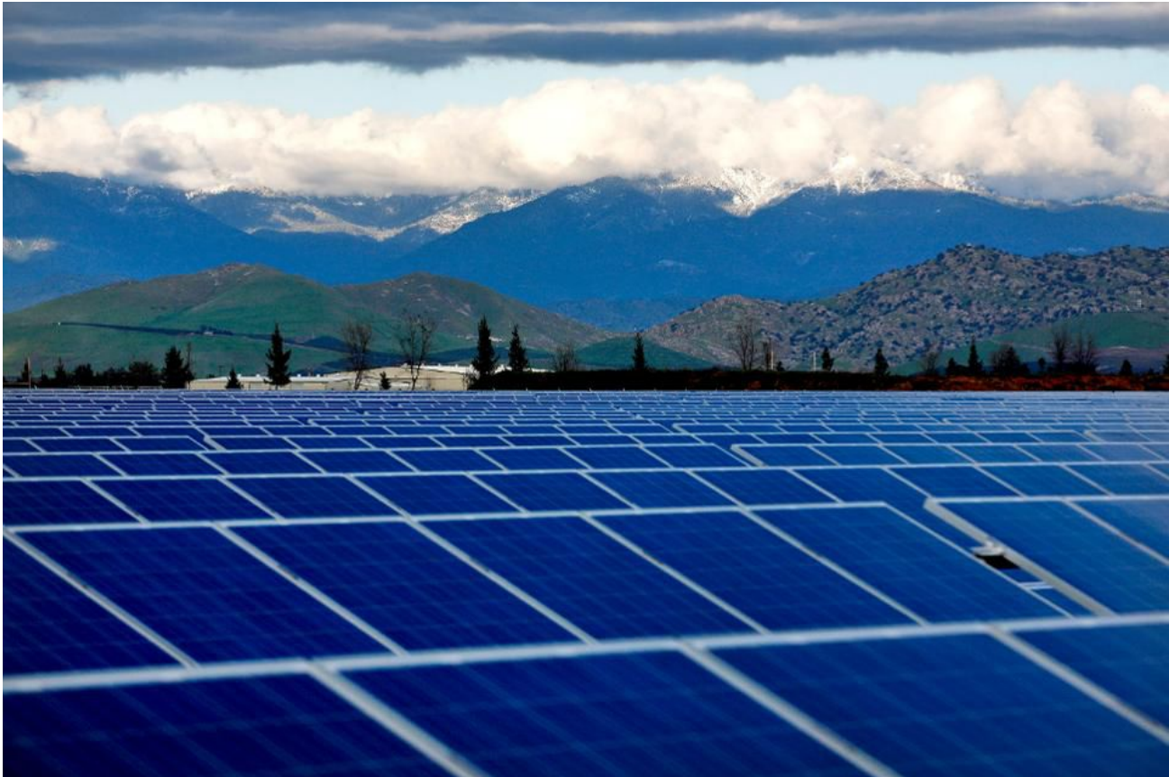
Mountains stand beyond solar modules at the Southern California Edison (SCE) solar array in Porterville, California, U.S., on Thursday, Feb. 17, 2011. Photographer: Ken James/Bloomberg
