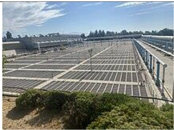
Sewage treatment at Tillman
