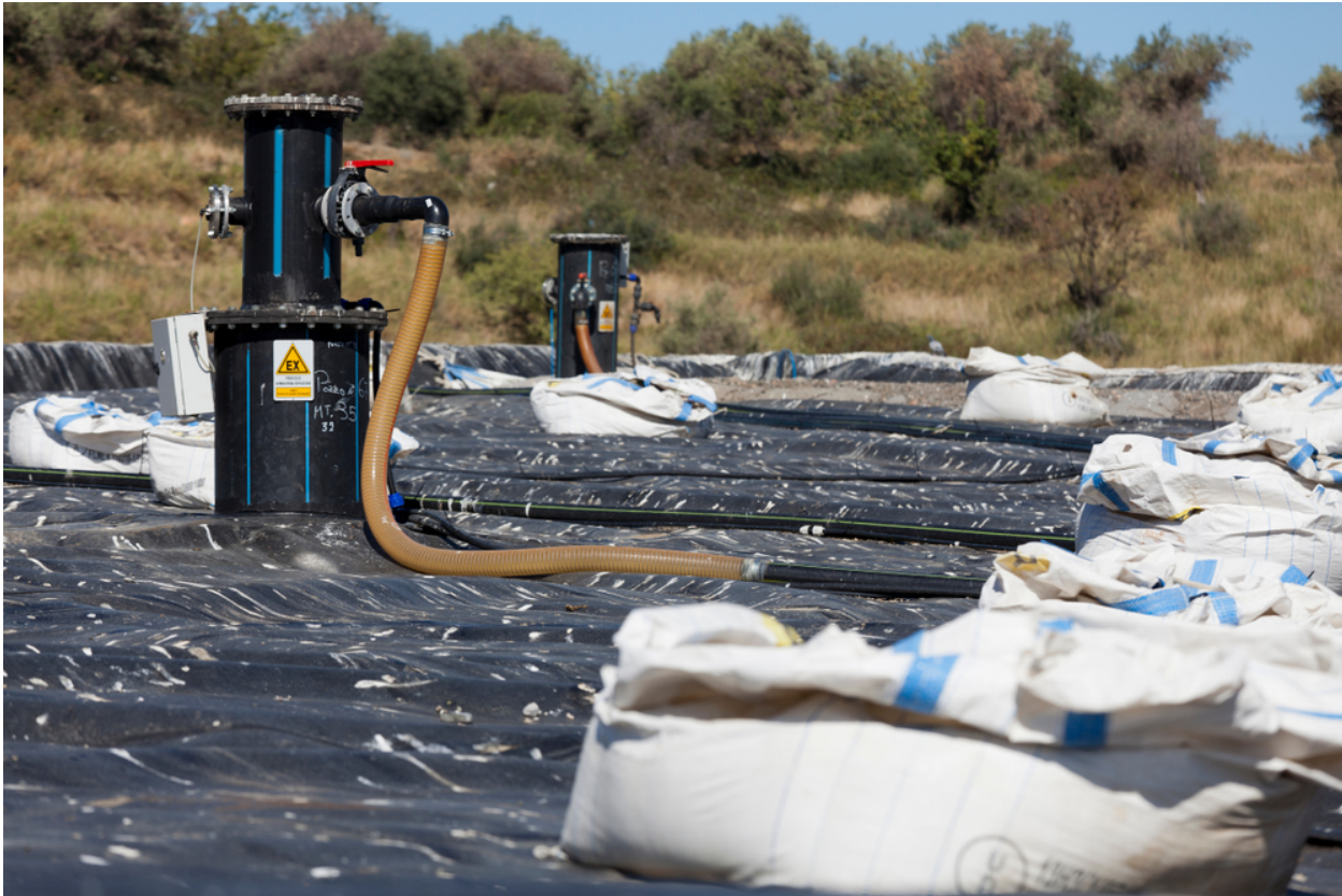
A landfill in Italy with a methane capture system. (Credit: newphotoservice/Shutterstock)
